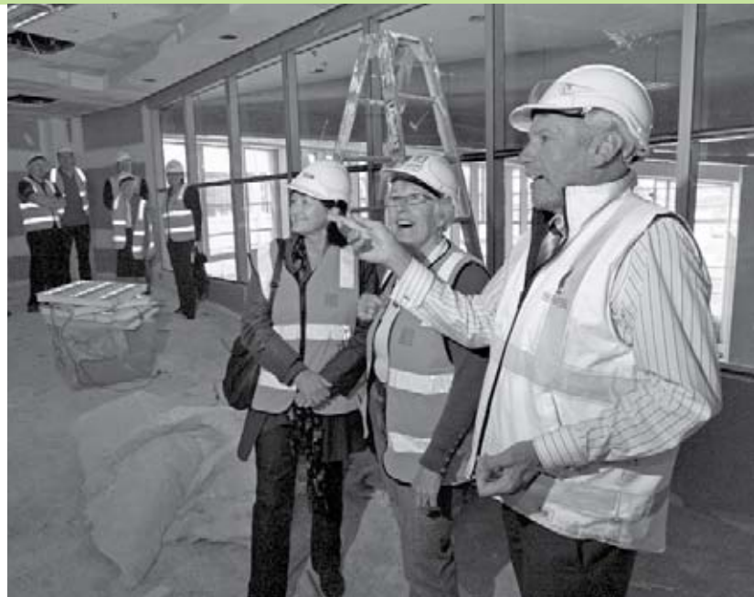
The enforced wearing of hard hats and high-visibility vests extended to the 300 VIPs Capital Redevelopment Manager Wayne Hall toured through our $115M Warrnambool Base Hospital construction site during 2010-11. Tour participants included our Woolsthorpe Auxiliary's Sue Sambell (left) and Wendy Ludeman. Photo courtesy of The Standard and photographer Aaron Sawall.
