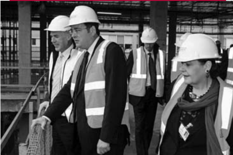
A Level-3 bird's eye view of the $115m construction site for (from left) SWH CEO John Krygger, Health Minister Daniel Andrews and SWH Chairman Sharon Muldoon.
