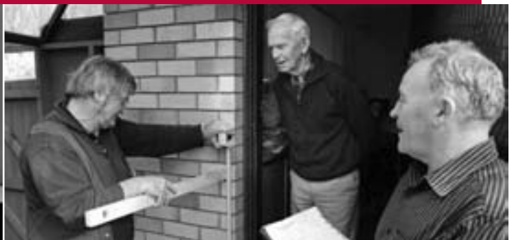
SWH Plumber James Moran and Occupational Therapy Assistant John Brooks are part of our Home Assessment Service that helps keep people safe by travelling as far as Camperdown, Timboon and Macarthur to install the likes of handrails, handheld showerheads and wheelchair-access ramps. Today it's Robert Tolley's turn.
