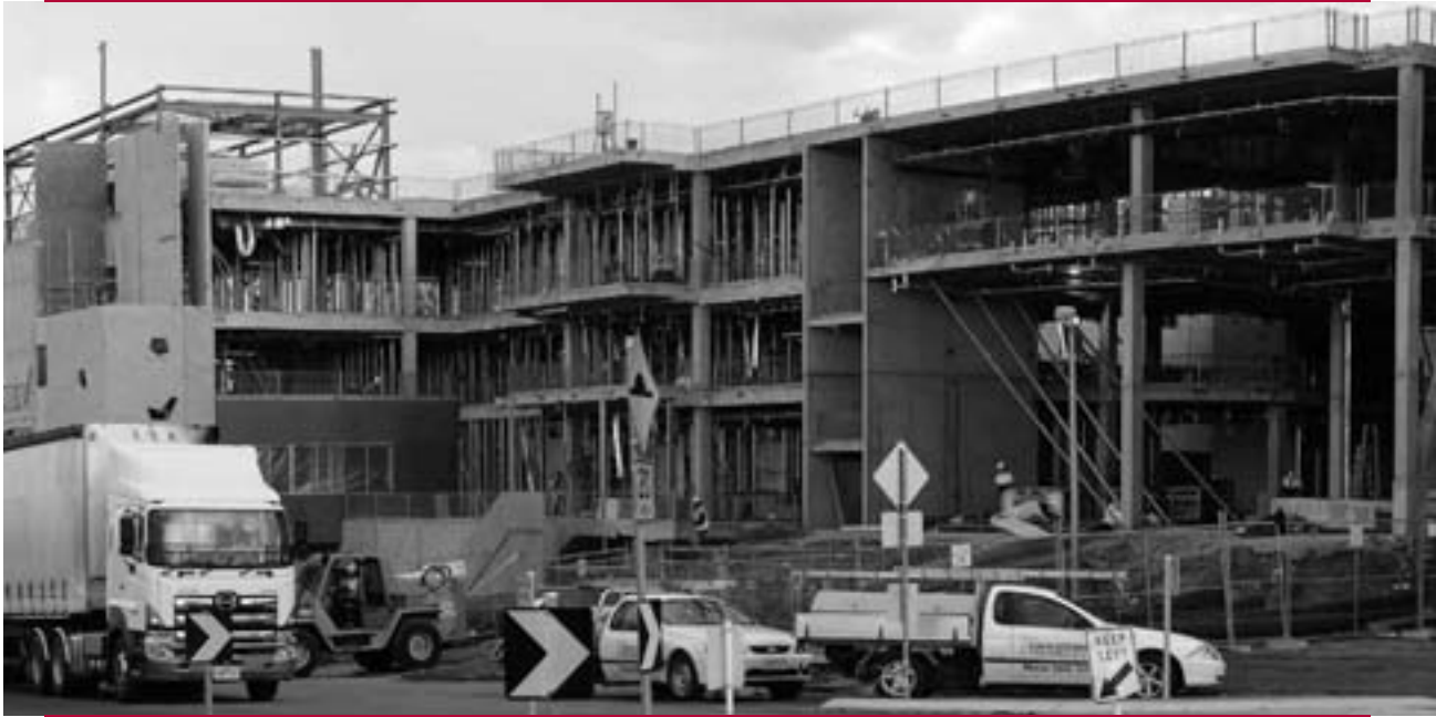
Our new Warrnambool Base Hospital will be amongst the most modern and technologically advanced health services in regional Australia.
