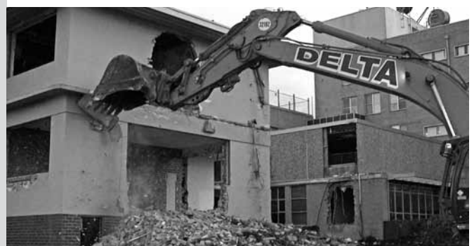
The demolition of Marcus Saltau House makes way for the $115 million capital project's greenfield site.
