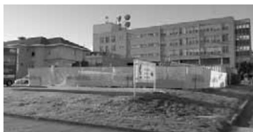
The redevelopment of the Warrnambool hospital has commenced with the work site set up.
